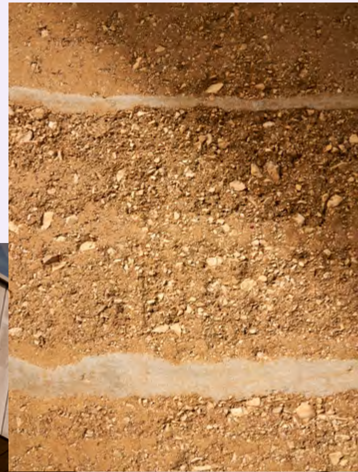
To construct the buildings, moist earth was layered into a slipform and mechanically compressed (rammed). Shell limestone was used for the lighter layers.
